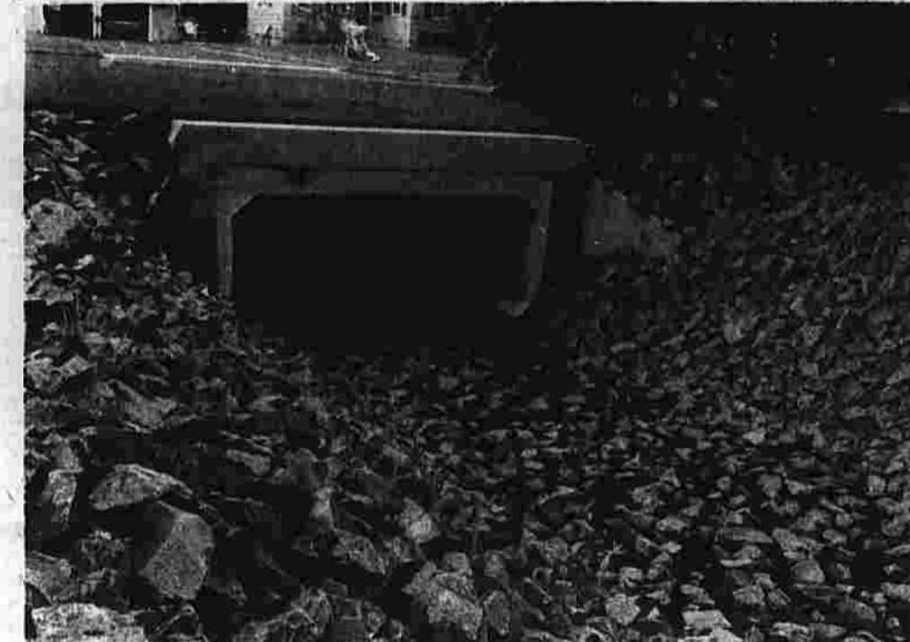
This culvert runs under a busy section of Forbes Street just before the intersection of Silver Lane. Before it was installed this year, residents of the area had a problem with flooding after heavy rain storms. But the
